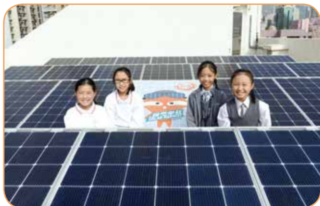
本局多間屬校於天台安裝了太陽能發電板。 Several of the affiliated schools of the Kuk installed solar panels on their rooftops.
